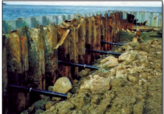
Project: San Clemente Island, Wilson Cove Pier Contractor: American Pacific Marine Location: San Diego, CA
