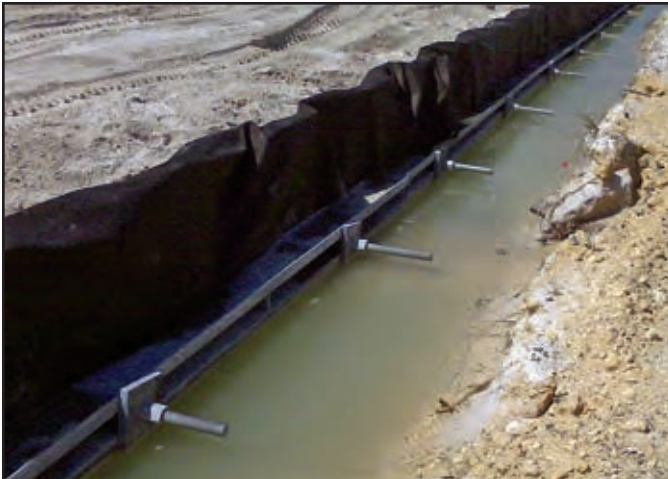
Project: Elgin Air Force Base Contractor: C.W. Roberts Contracting & Contech Construction Products Location: Destin, FL
